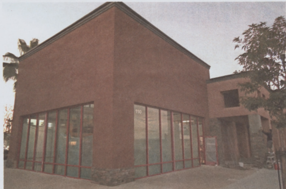
The façade of the under-construction El Cajon Brewing Co. on the corner of N Magnolia & Main in El Cajon
